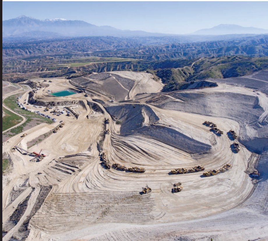
Sukut Construction ( No. 313 ) moves 2 million cu yd of material at a landfill excavation project in Redlands, Calif. Construction includes a desilting basin, two engineered stockpiles, 17 acres of composite geo-membrane liner, leachate collection and a stormwater system and paved haul road.
